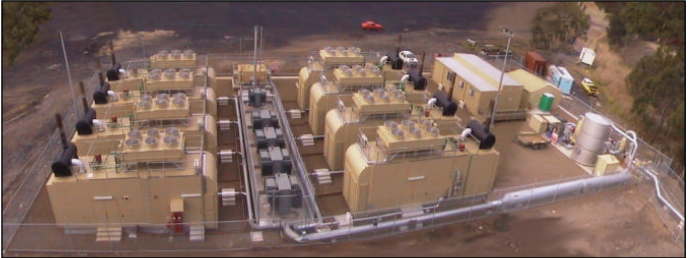
Clarke Energy turnkey supply of 8 x 1MWe GE Jenbacher JGS 320 GS-S.L
