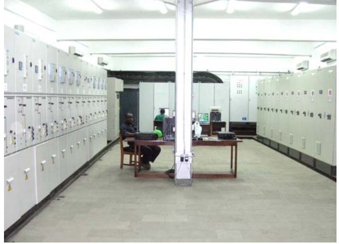
Flour Mills control room
