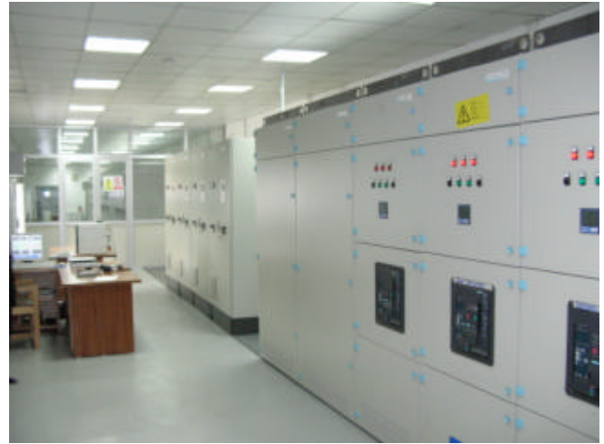
Bagco generator control room
