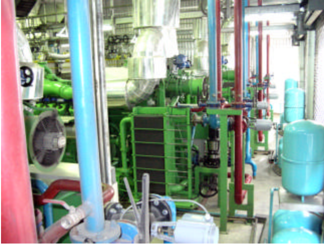
Bagco generator room
