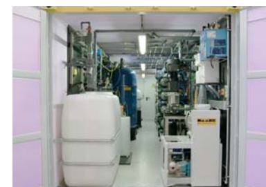
Reverse Osmosis leachate treatment containerised installation
